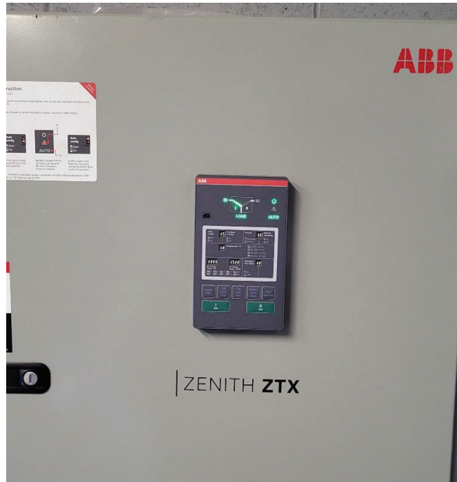
Figure 3-1: Sativa Well-3 Existing Automatic Transfer Switch
