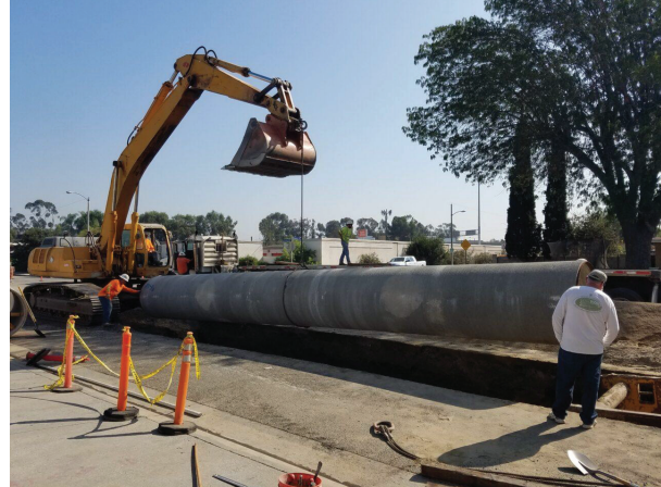
Installing the 48-inch M-Line, the main delivery pipeline that provides water for all Company shareholders.
